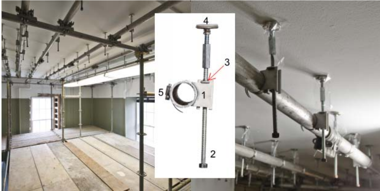
Figure 2: The Temporary Plaster Support System Deployed at the Colonial Building in St. John's, Newfoundland, summer 2011.
